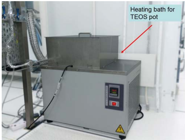
Fig. 2b: The heating bath for TEOS pot located at the rear of the main machine.
